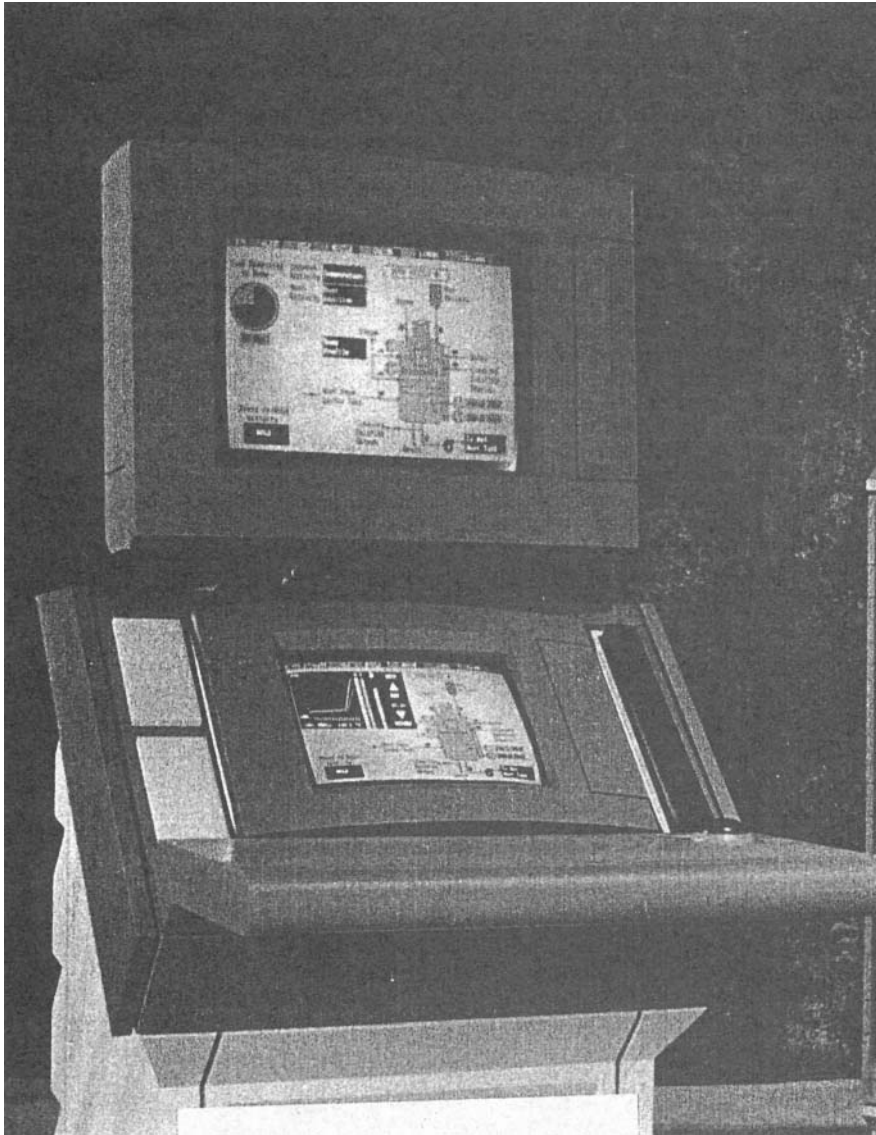
Figure 14.5(b) Control panel and display of Foxboro Intelligent Automation computer system (Foxboro Company Ltd)
