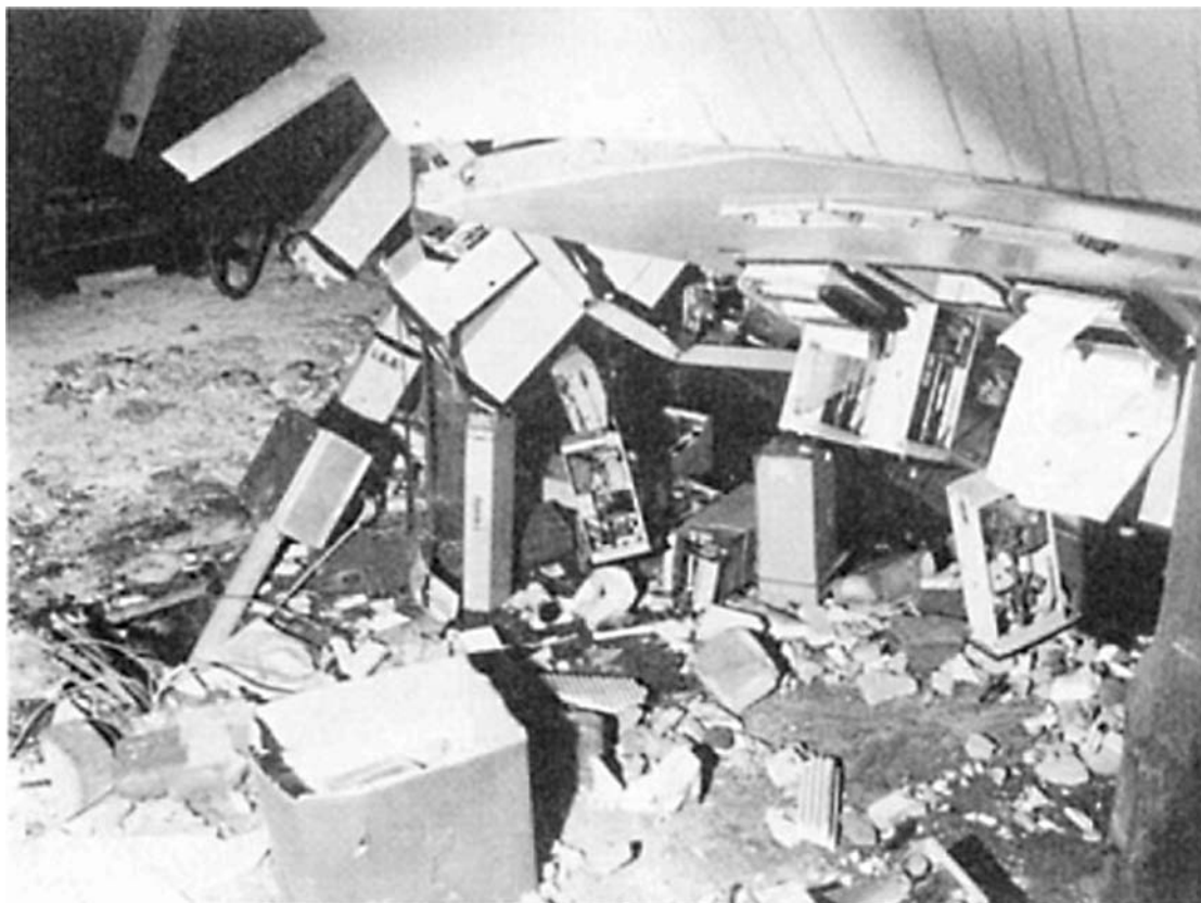
Figure A1.13 Seek, 1975: damage to instrumentation in the control room (Ministry of Social Affairs, 1976)
