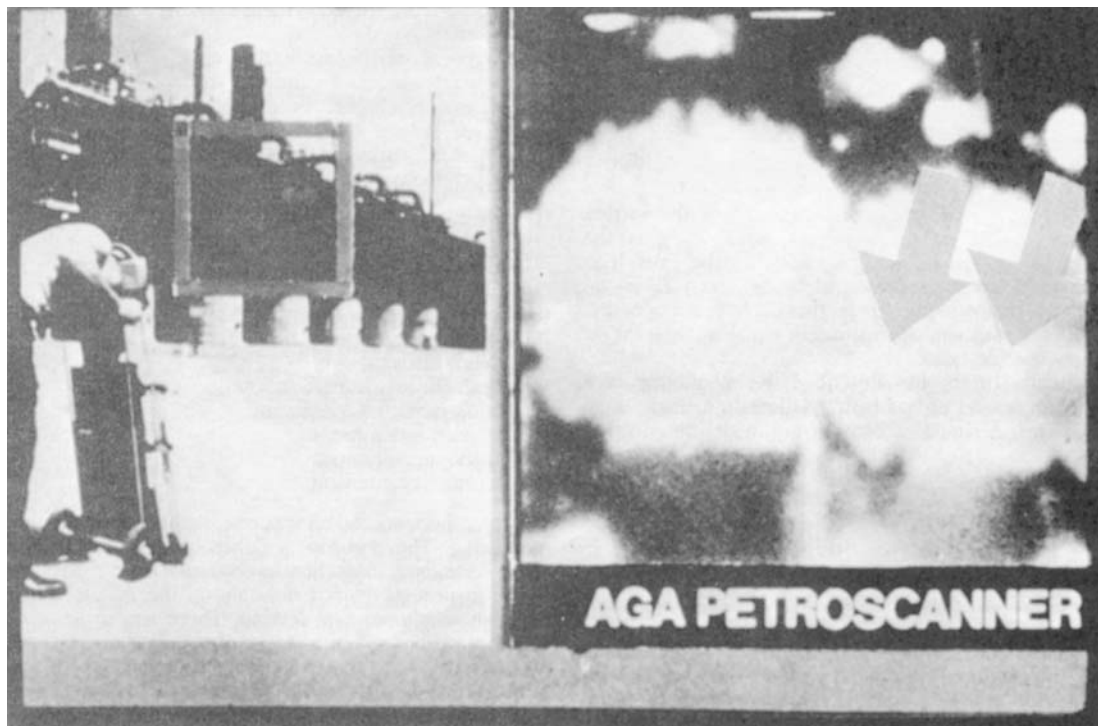
Figure 19.4 Normal and thermographic photographs of a refractory lined vessel (A GA Ltd): (a) normal photograph; (b) thermographic photograph, with arrows indicating thin spots
